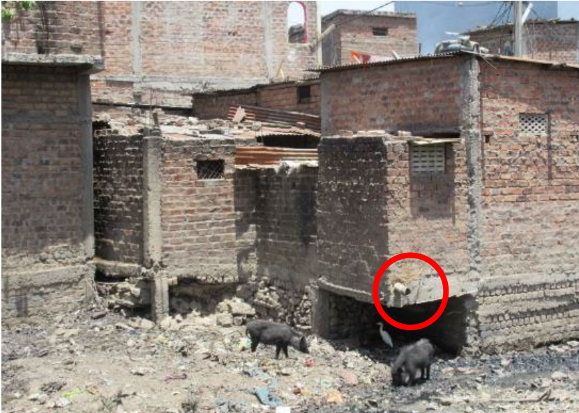
Toilet flowing out behind house
