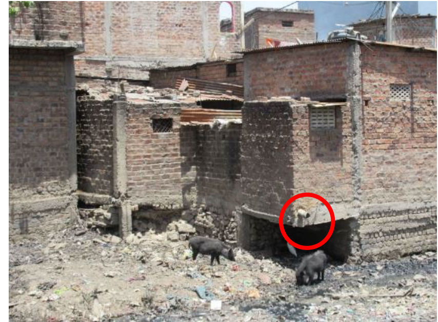
Toilet flowing out behind house
