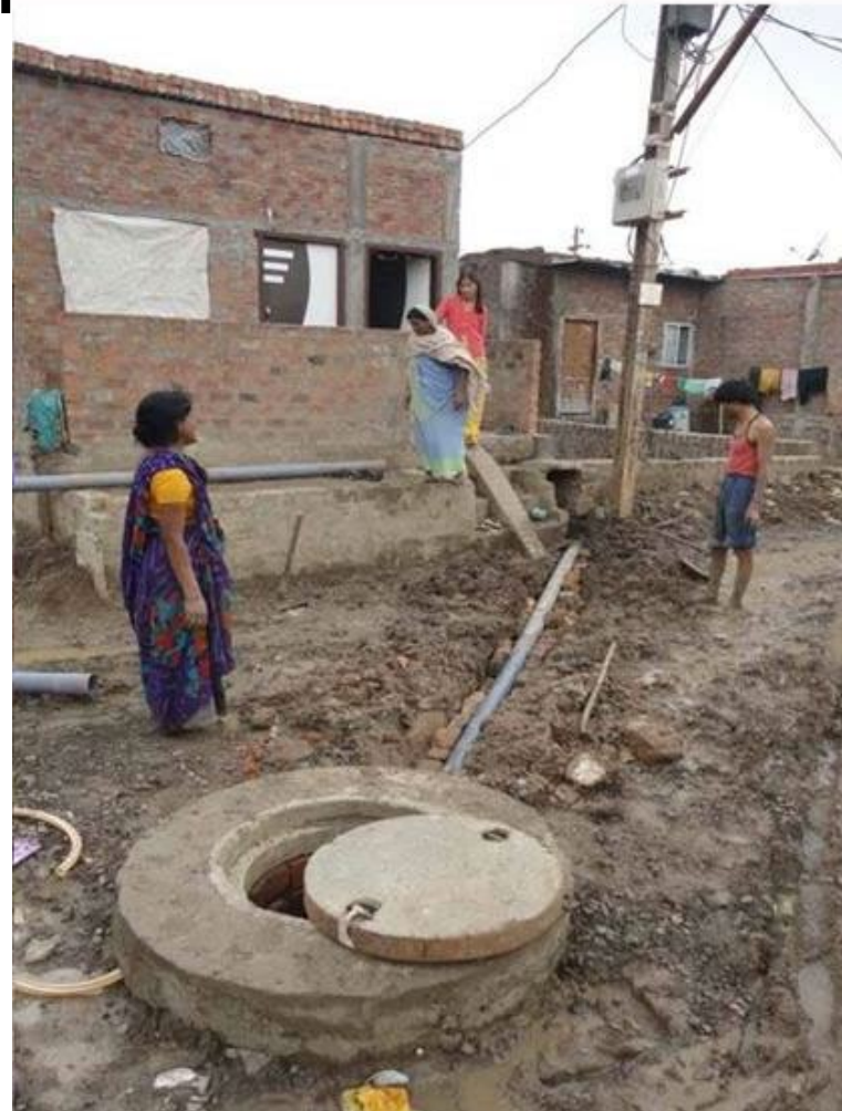
Sewerage system being installed in slum and sewerage pipe being connected to toilet
